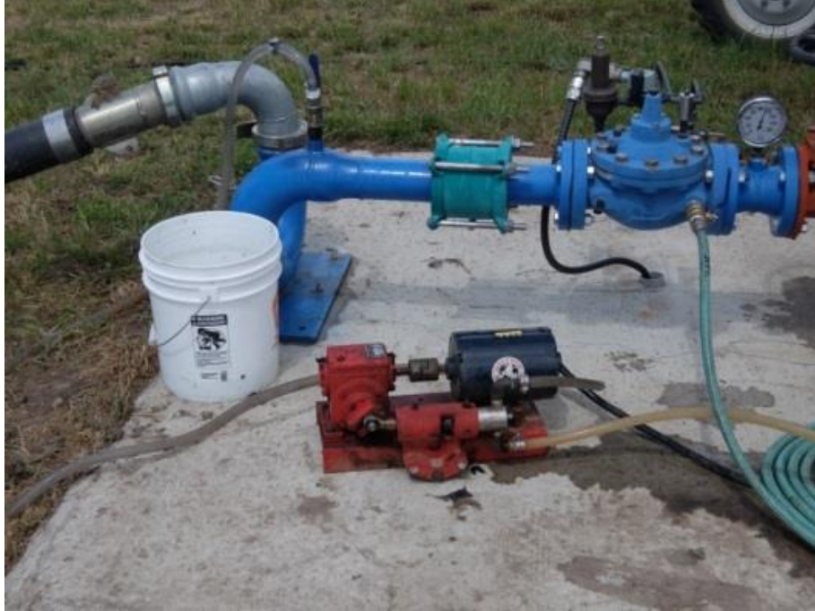
Figure 31. Solution fertilizer injection apparatus ( Inject-O-Meter piston pump).
